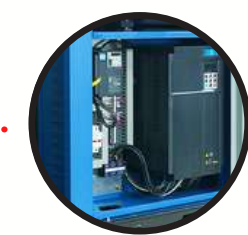
VSD Controller for Main & Fan Motor
